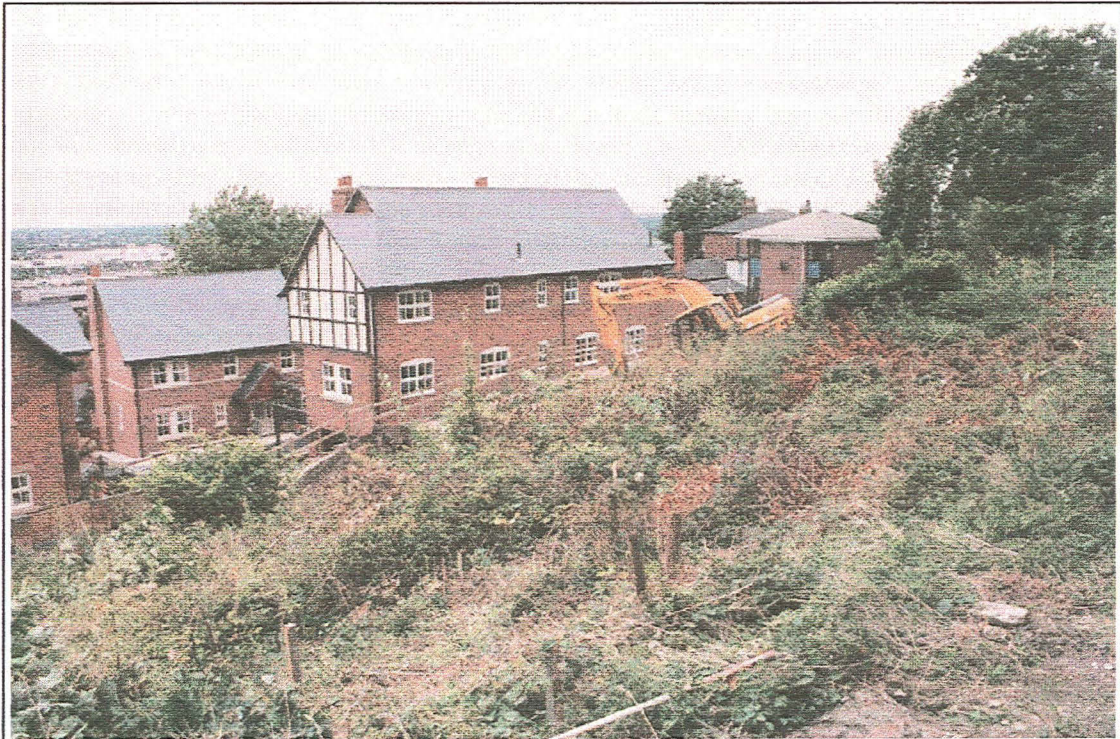
Plate 1: General view of the site looking south-west towards Stanthaket Court prior to the excavation and formation of terracing for Plots 1 & 2.
