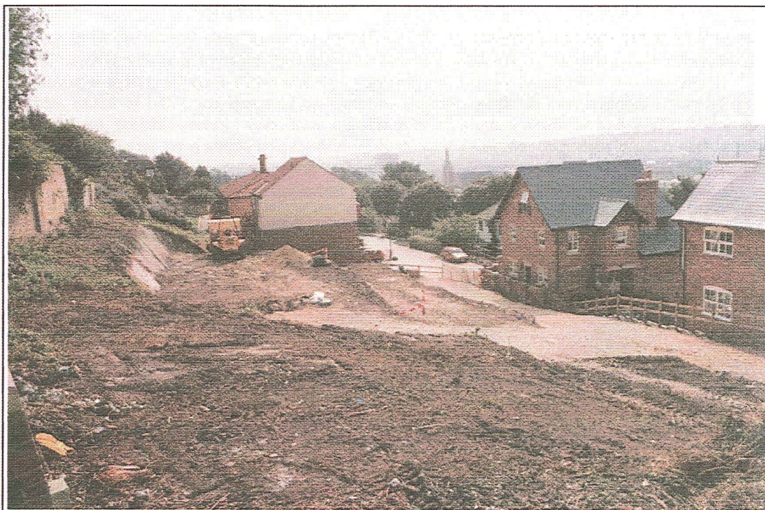
Plate II: View of site after terracing (looking south-east). Although extensive, little damage was caused to the buried archaeology, the majority already having been lost during the construction of terraced housing on the site during the Victorian period.
