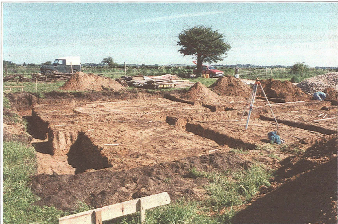
Plate 1: General view, looking north, of the foundation trenches for the new dwelling. Note the minimal topsoil coverage above the pale brown natural sand.
