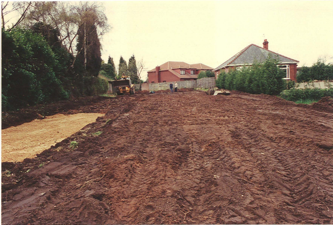
Pl. 1 The development site, looking west: the foundation trenches are located at the rear of the plot
