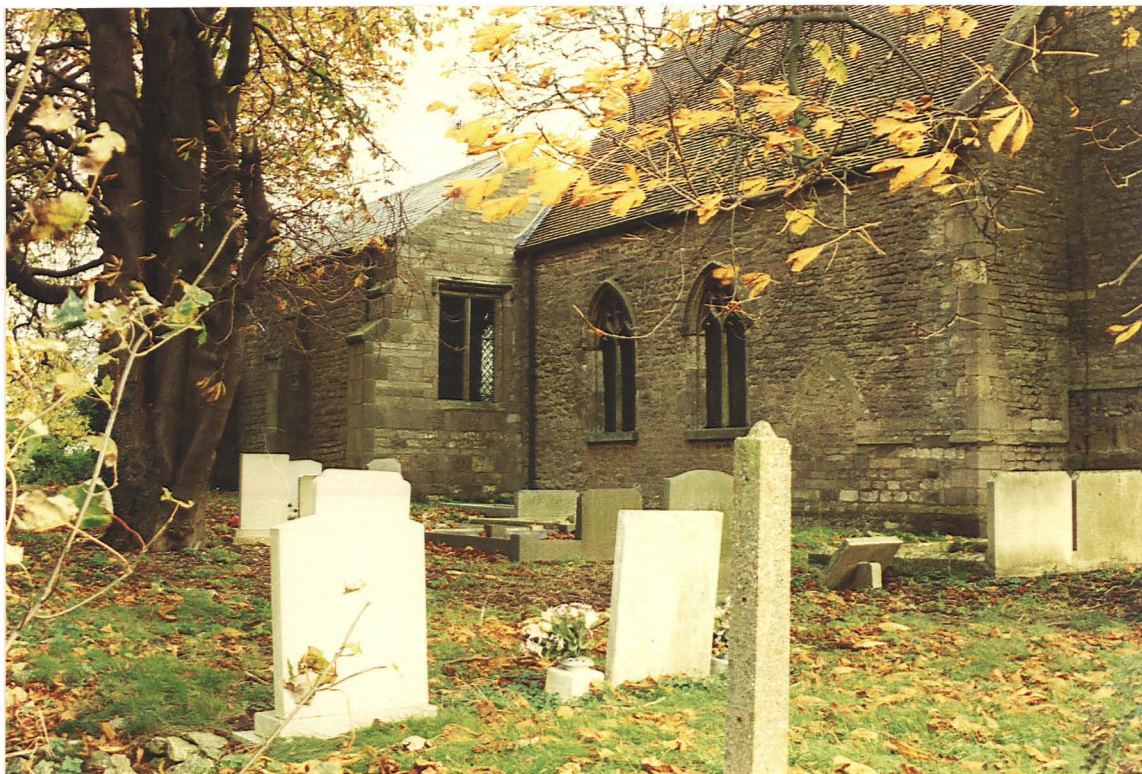
Pl. 12 Opening 1 clearly visible in the wall face
