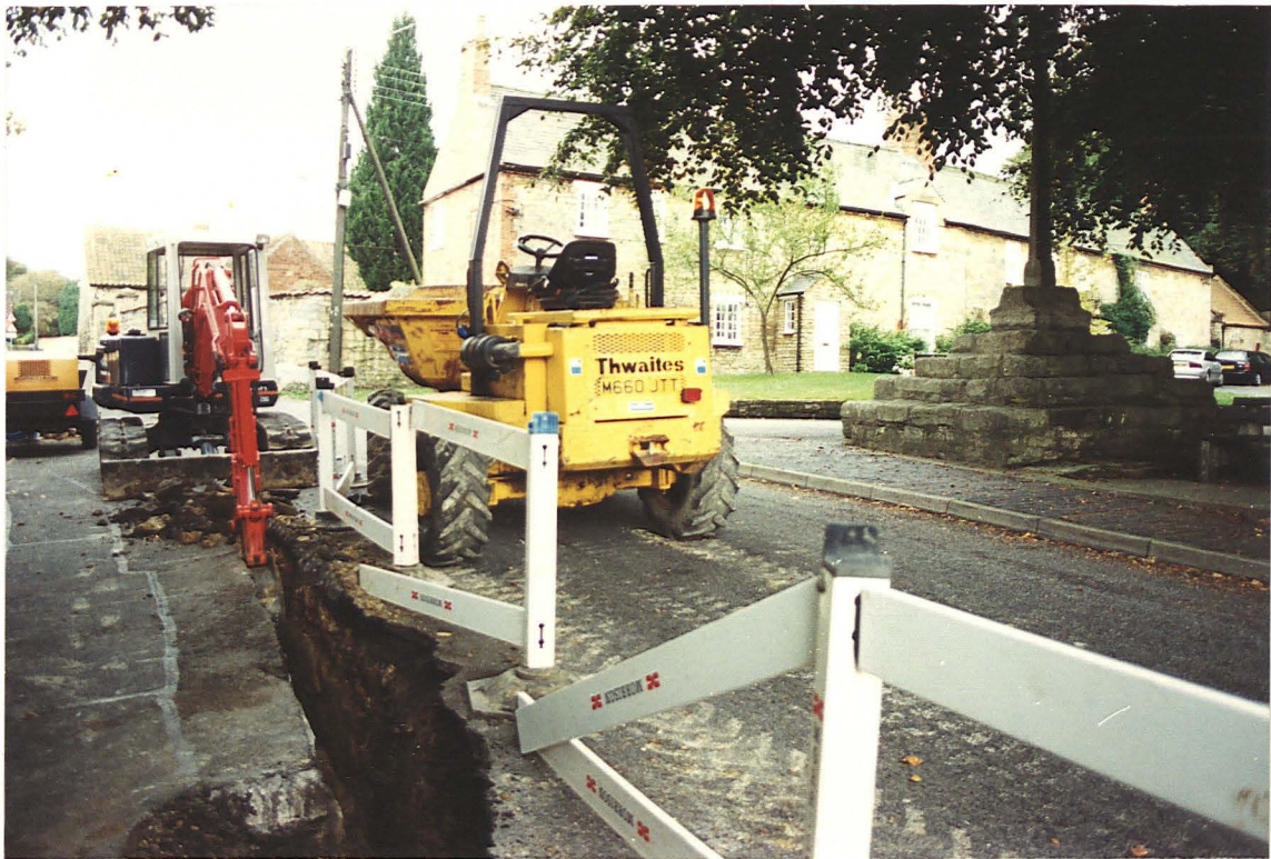
Pl. 18 Trenching at 6a, opposite the medieval cross base, High Street, Washingborough (looking south).
