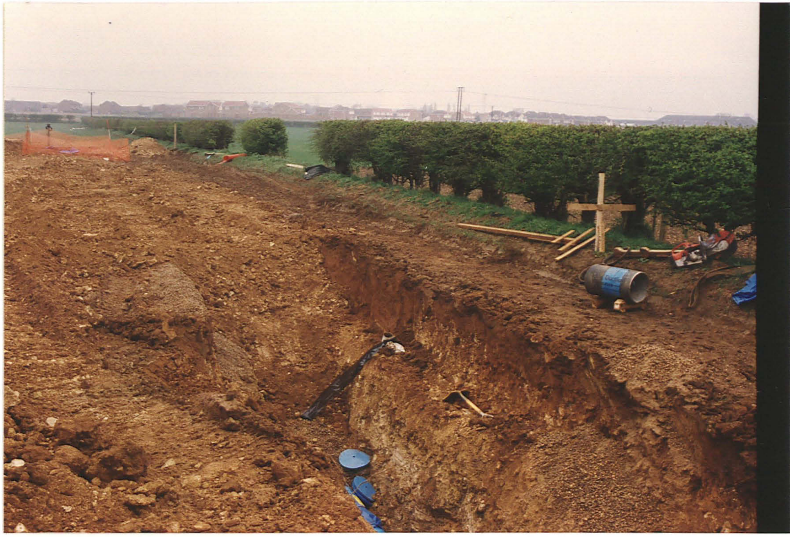
Pi. 10 Partly backfilled pipe trench alongside the parish boundary, Field 1. The dark brown loam in the trench side is subsoil and the fill of archaeological feature 1H. Looking NE.
