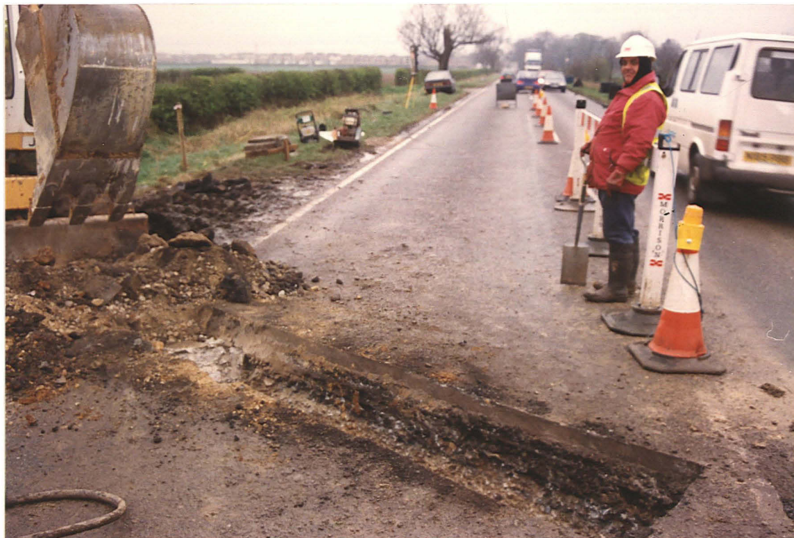
Pl. 15 Excavation of the pipe trench across the western side of Sleaford Road. The fine rounded gravel of the Roman road surface is visible below the tarmac. Looking north.
