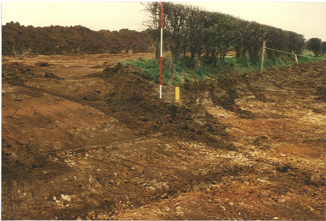
Pl. 12 Field boundary between Fields 1 and 2. Note the difference in ground height, and the presence of spread loam subsoil in Field 1. (Looking NW from Field 2).
