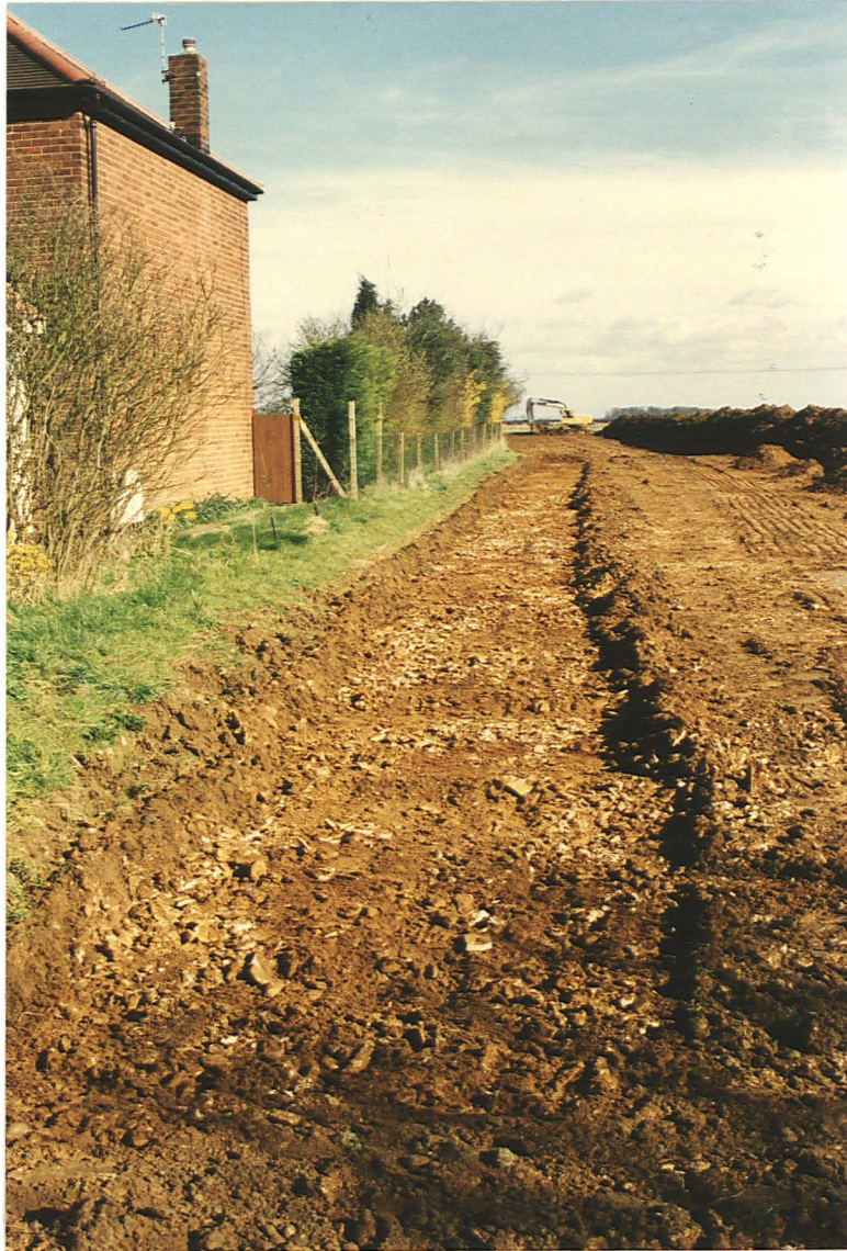
Pl. 2 Field 1: Part of the stripped easement was scraped by machine to try to reveal the Roman road. Looking east from Grantham Road.
