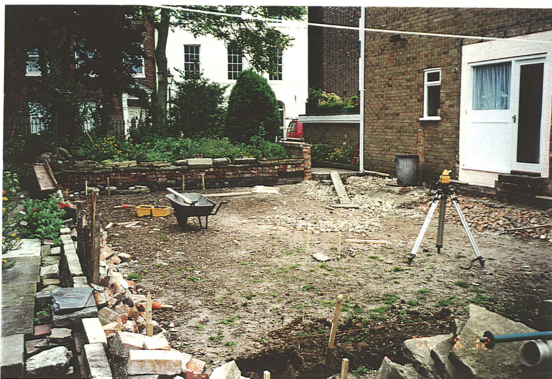
Plate 1: General view of the site, looking north-east toward the Georgian houses on the eastern side of Witham Place.
