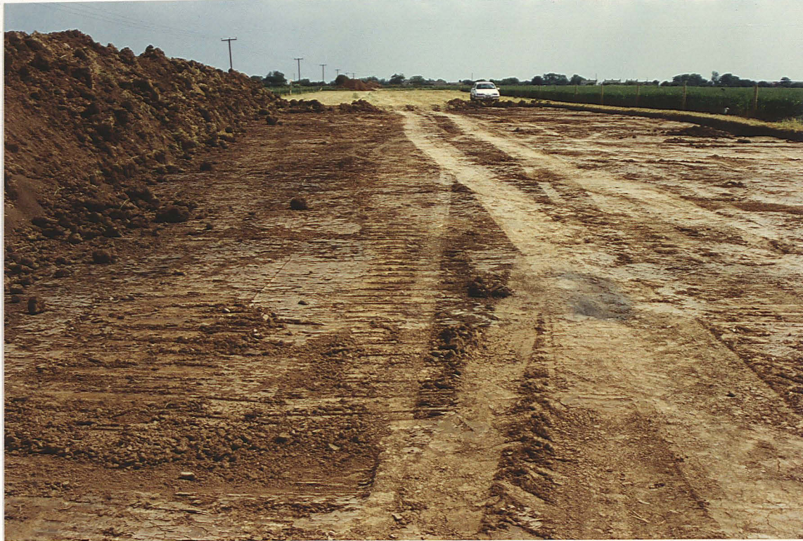
Pl. 5 Multiple unexcavated features similar to 10A, containing ash, were seen across this section of easement after topsoil removal. Looking SE from northern end of Field 10, with 10A on right edge of the easement.
