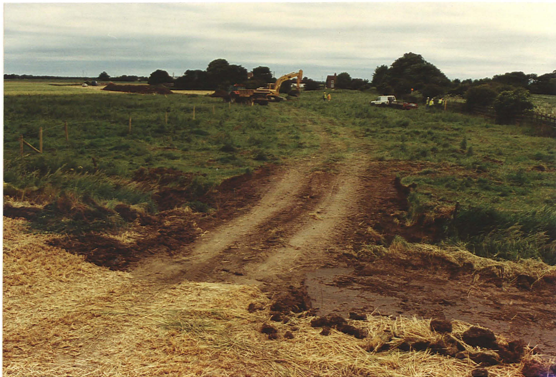
Pl. 17 Clearing the pipeline easement in Fields 18 and 19, north of Theddlethorpe All Saints (looking south across ridge and furrow, with the railway line to the right).
