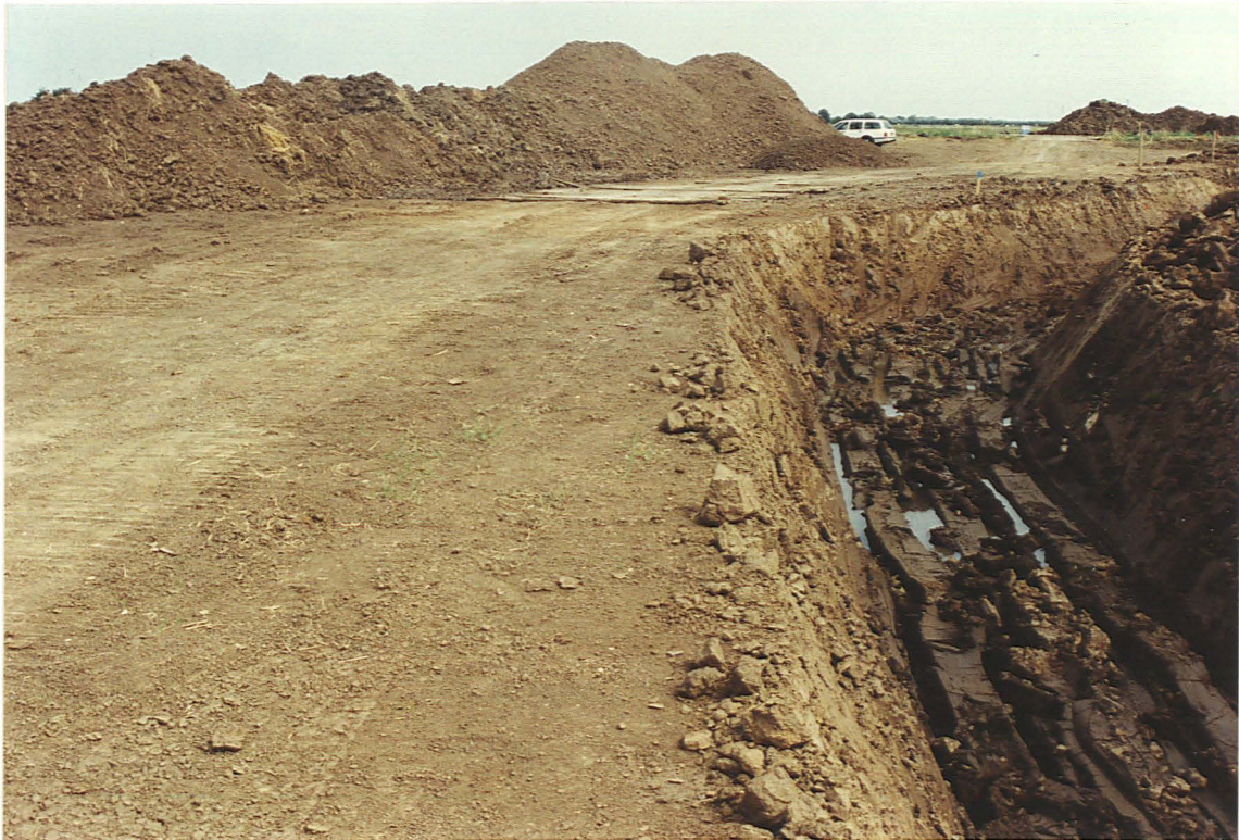
Pl. 14 Planking protecting Excavation Area B, with the pipe trench in Field 17. The white stones in the trench side mark a backfilled field ditch. Looking SW.
