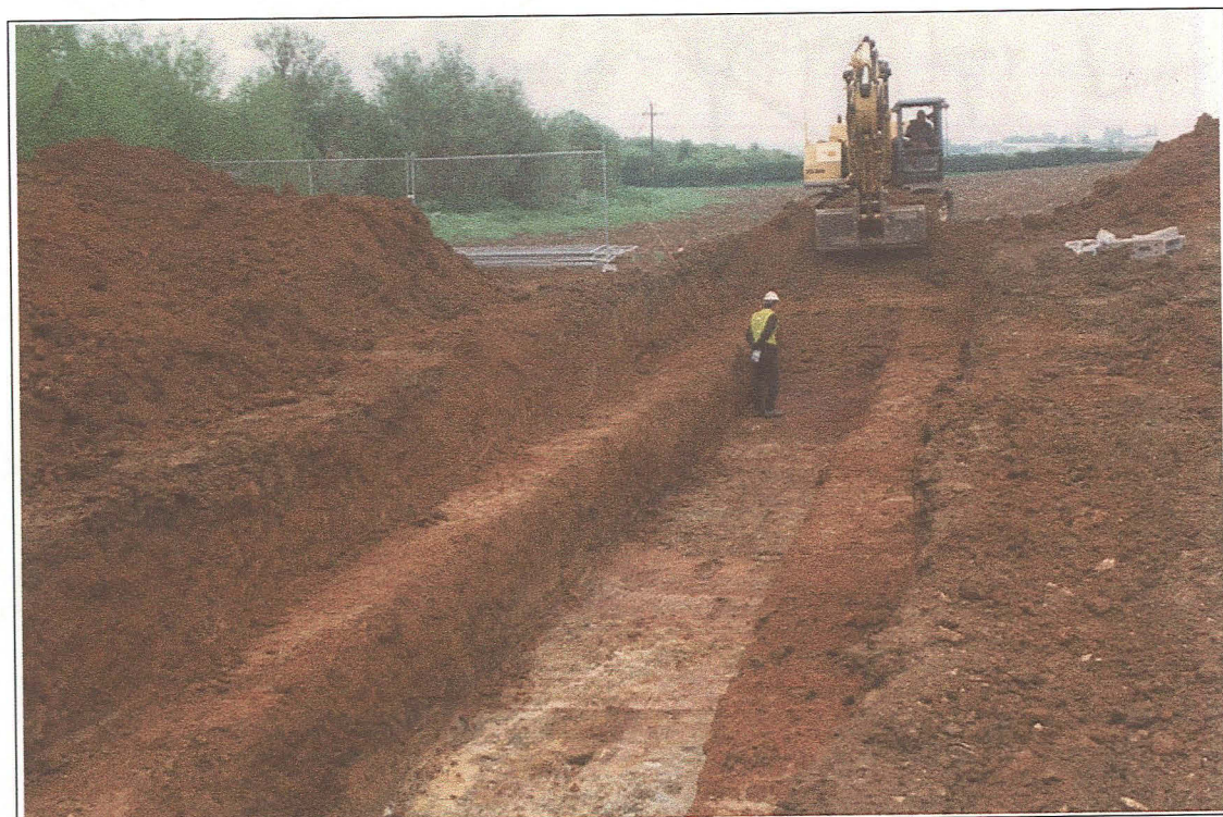
Plate 6 - Removal of colluvium by machine in Trench 8 - work in progress, looking south-west
