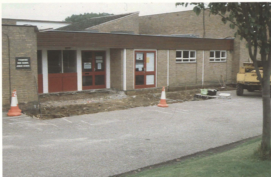
Plate 1 General view of area of excavation, looking west towards the existing school porch
