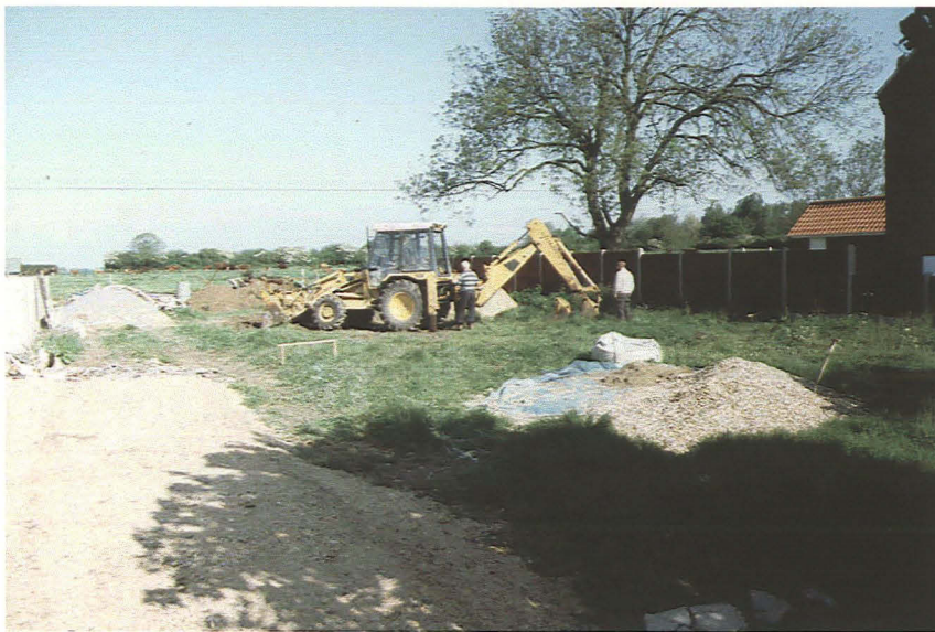
Plate 1 General view of the site prior to commencement of groundworks, looking northwest
