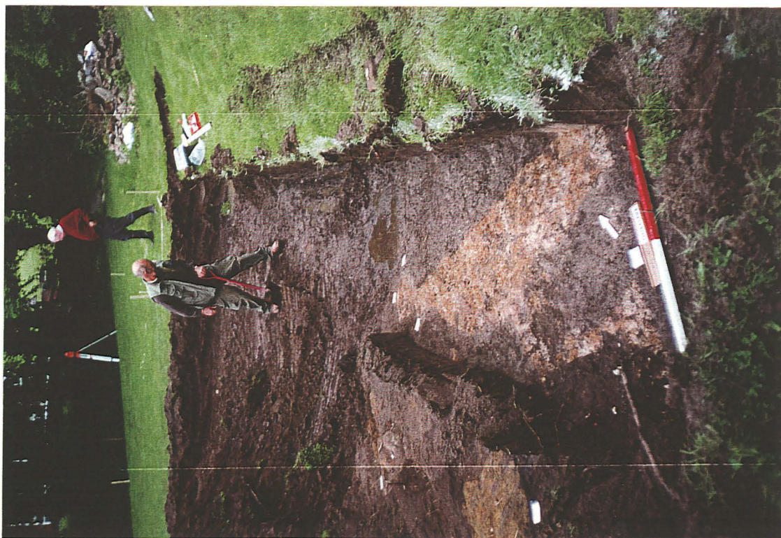
Plate 2: The complex of features exposed along the eastern edge of the building footprint, looking north.
