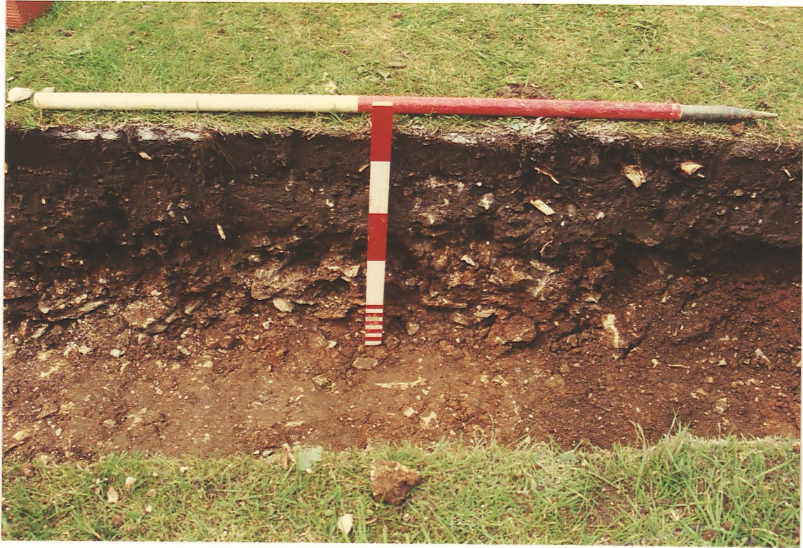
Pl. 3 Section through excavated foundation trench, looking west (0.50m vertical scale and 1m horizontal scale)
