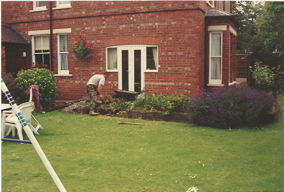
Pl. 1 The development site prior to the excavation of the trenches, looking east
