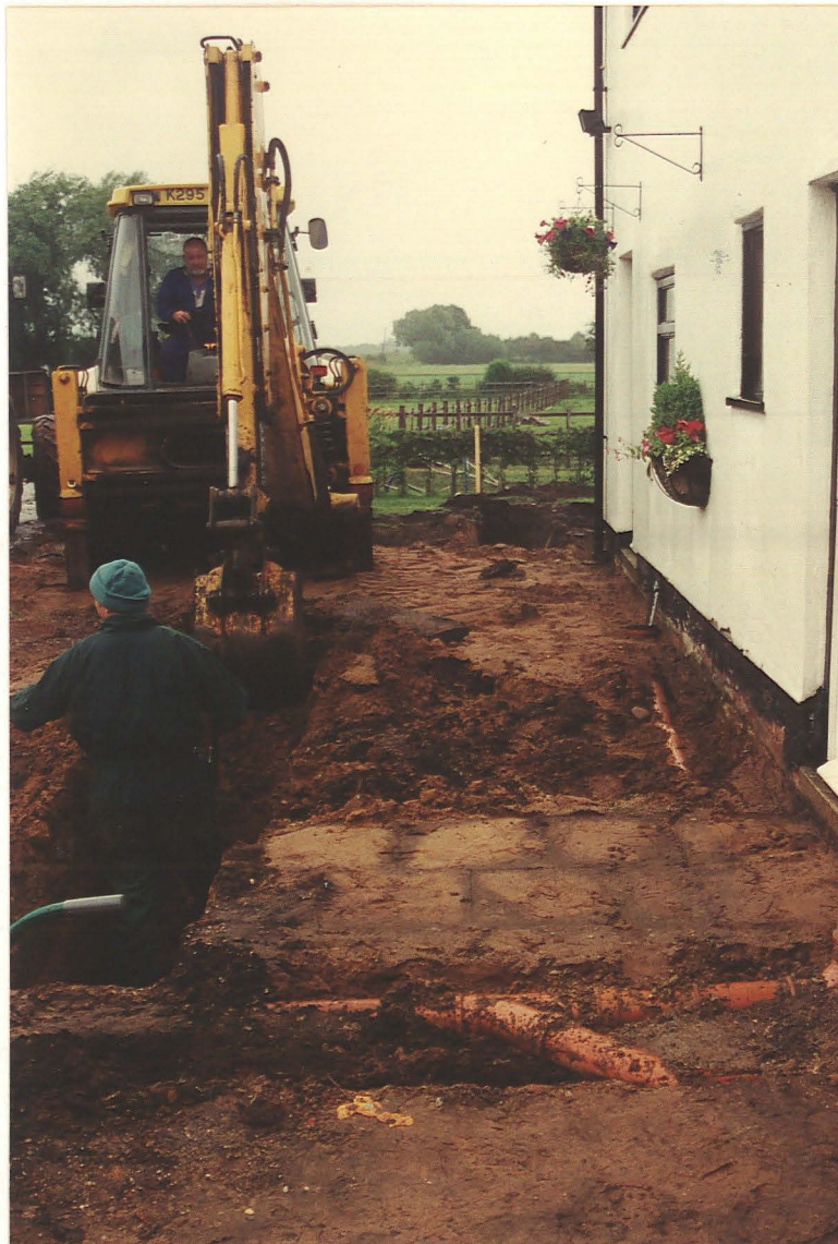
Pl. 4 Disturbed ground and waste pipe in the foundation trenches in front of the existing farmhouse
