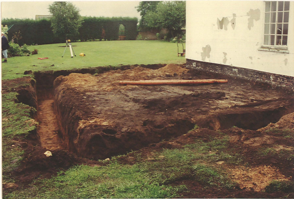
Pl. 1 Foundation trenches for the two-storey extension adjacent to the existing farmhouse, looking south
