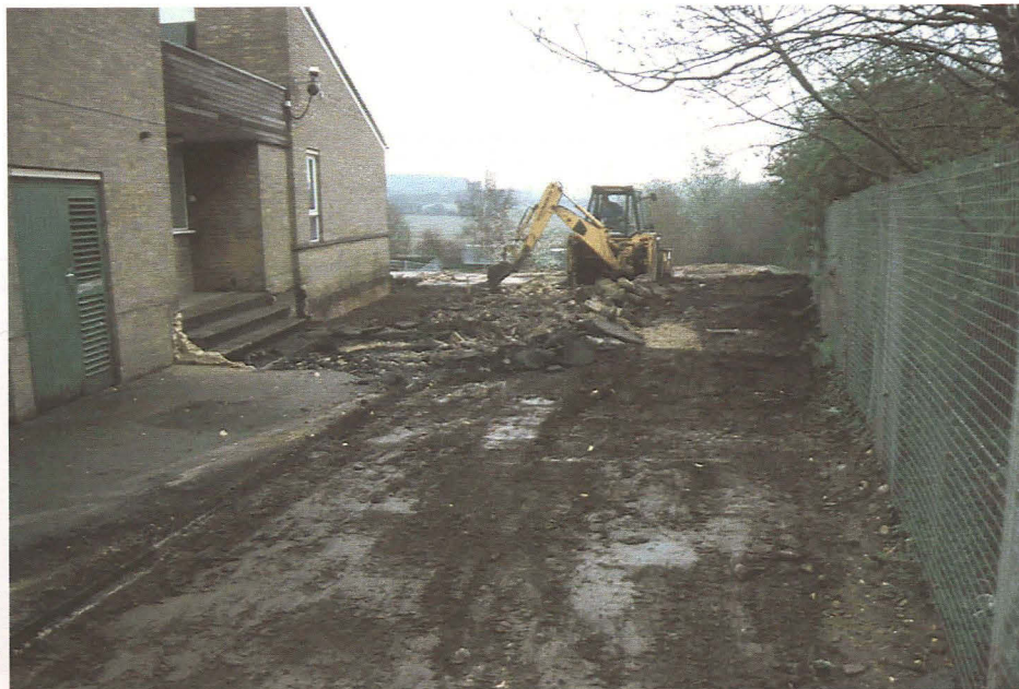
Plate 2 General view of stripping in preparation for the raft, north of the school
