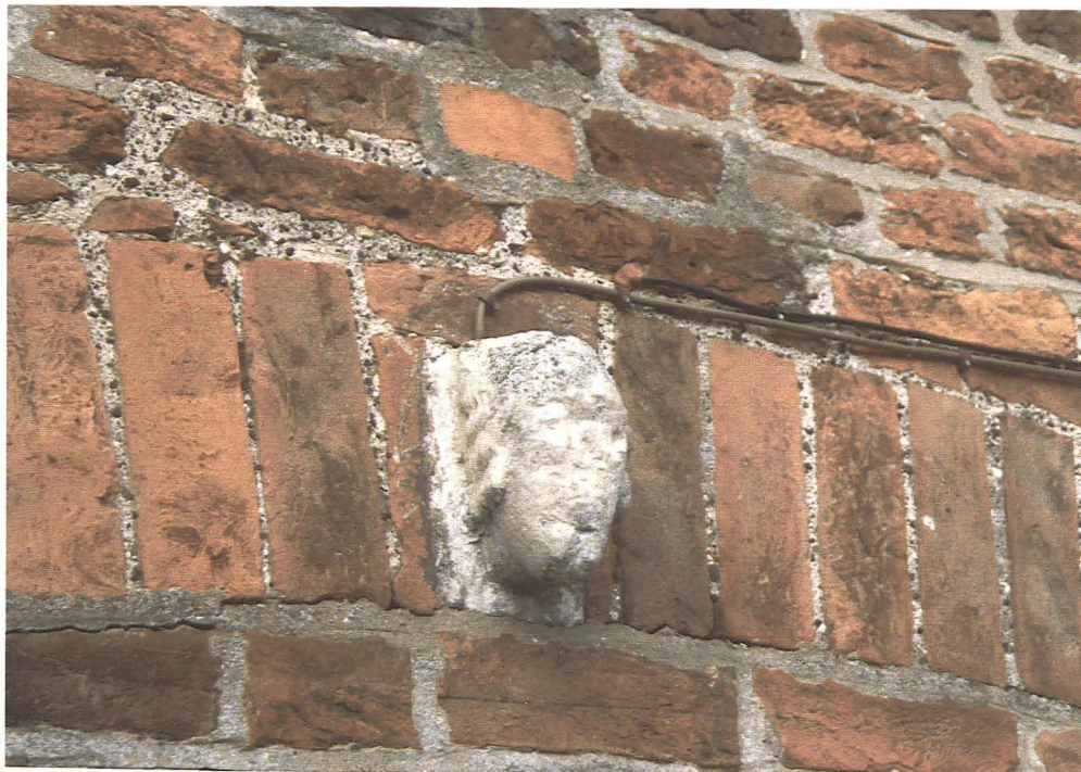
Plate 4 Re-used medieval stone head corbel in east wall of the existing building
