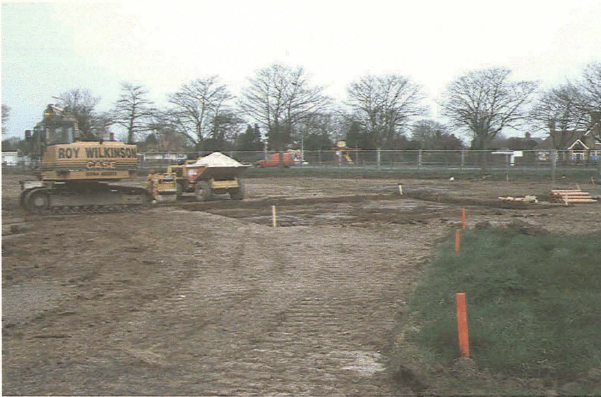
Plate 1 General view of the development area looking northwest, showing an excavated raft foundation
