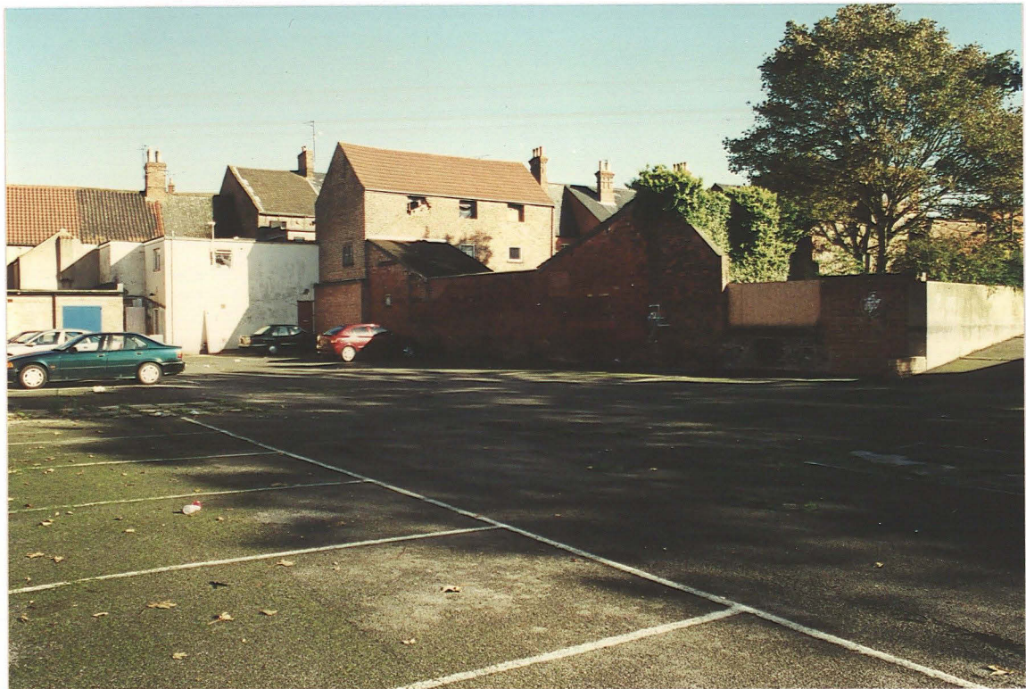
Pl. 8 Brick boundary wall and ramp to adjoining land, east of the yard area (looking NE).
