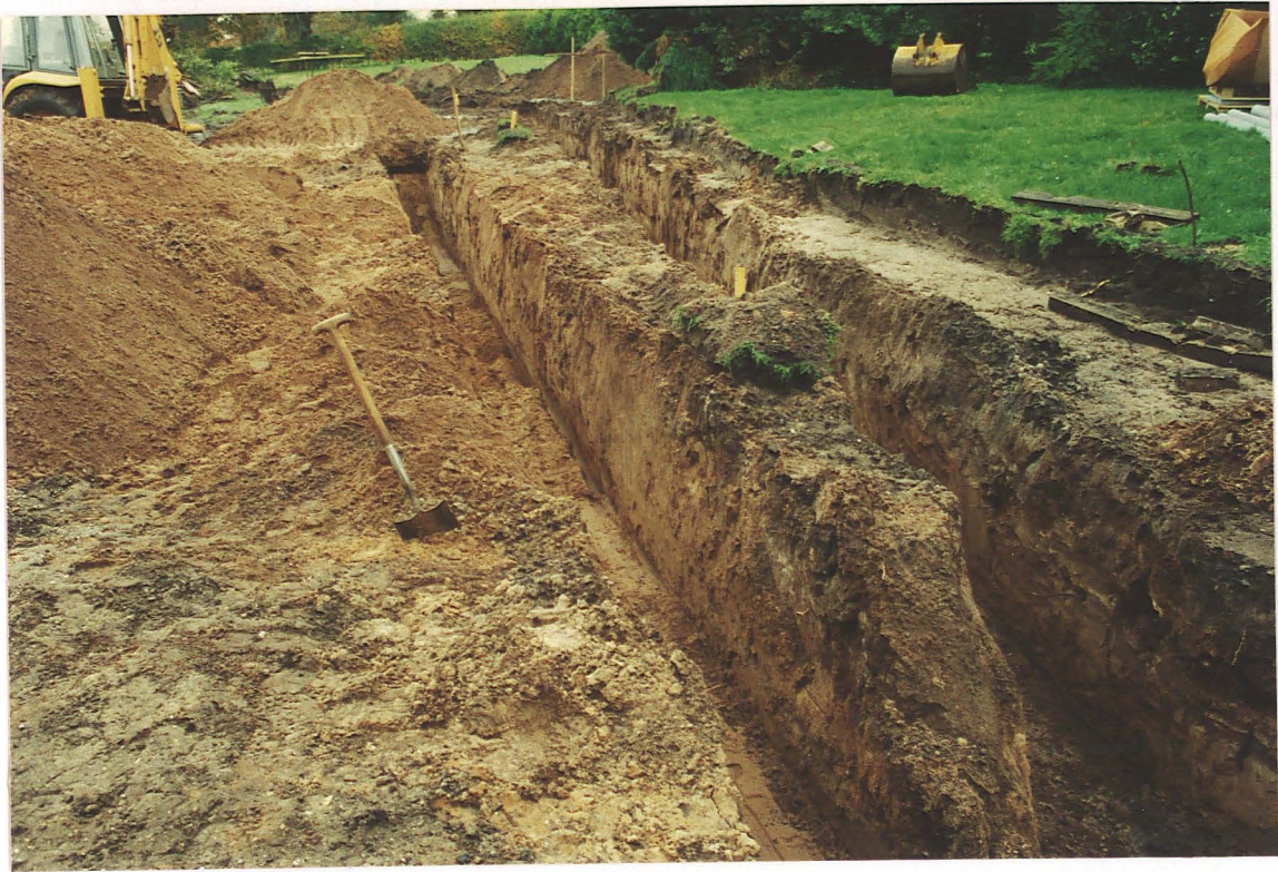
PI. 7 Central part of the access road showing area showing two drainage trenches.
