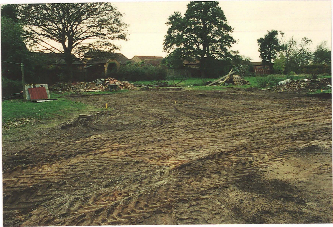
PI. 3 Western part of the access road, top centre of the picture shows gravel area, looking west.
