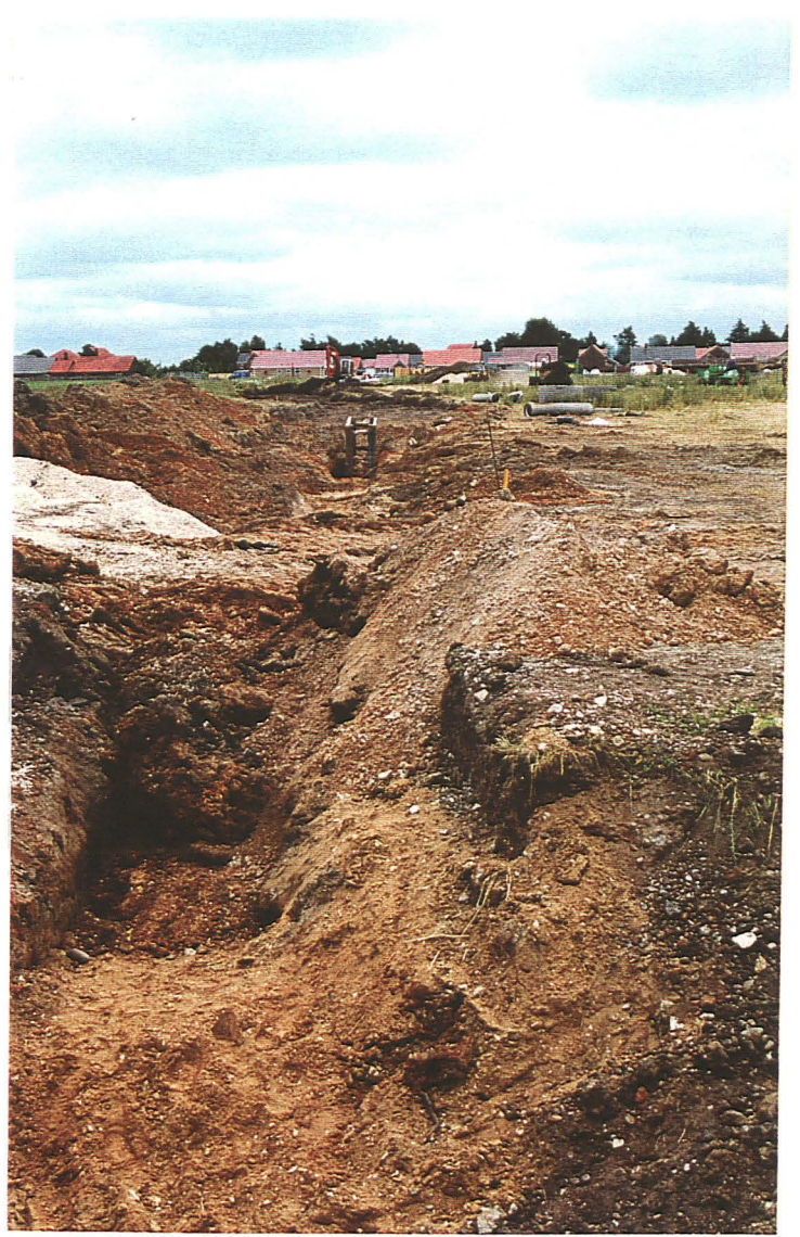
P7. Looking south from Green Lane along main sewer and access cut
