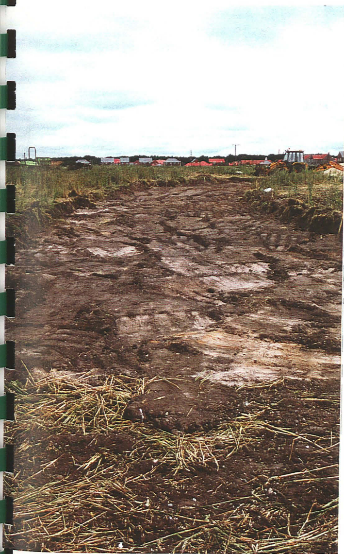
P6. West access road strip in Phase II area (southernmost), looking east
