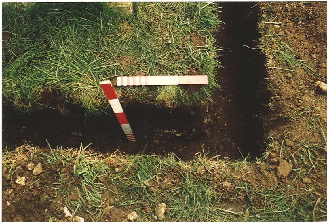
Pl. 8 Chalk rubble foundation for NW tower buttress, exposed beneath the turf (looking south; vertical scale 0.5m, horizontal 0.3m).
