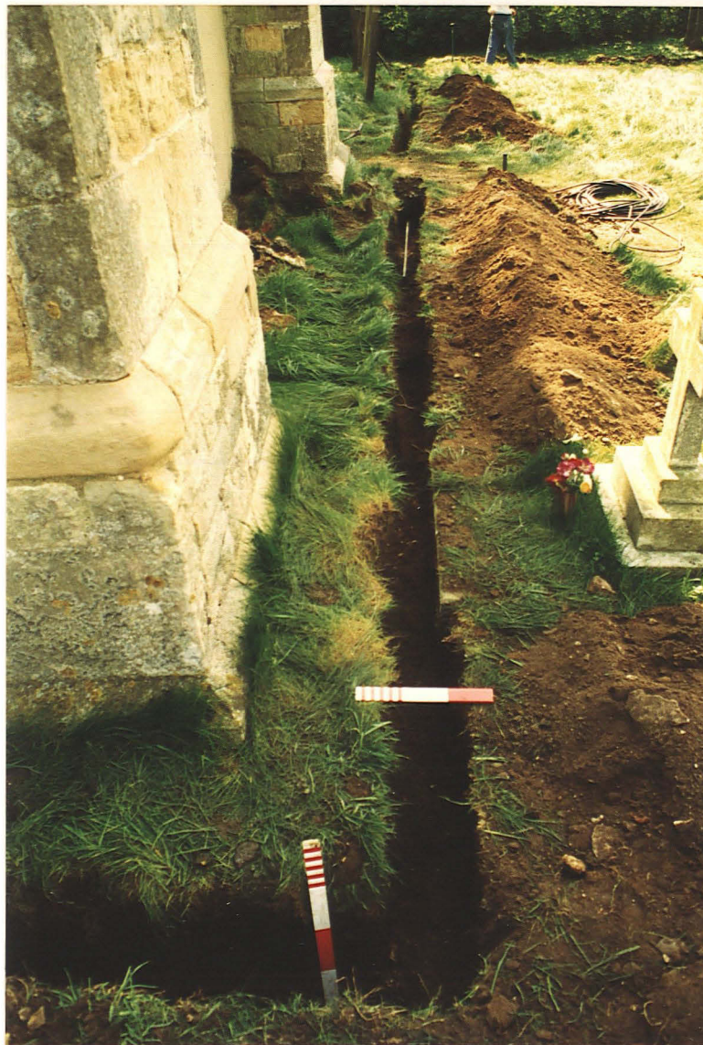
Pl. 7 Service along the west side of the church (looking south; vertical scale 0.5m, horizontal 0.3m).
