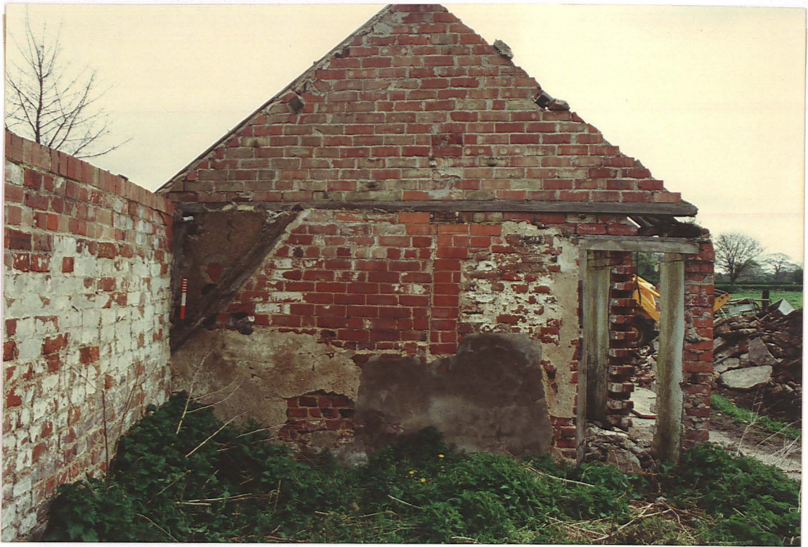
Pl. 9 Cross wall at west end of cattle shed showing remains of mud and stud wall
