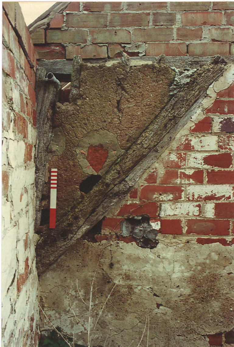
Pl. 10 Close up of brace and cross frame fragment belonging to a mud and stud building
