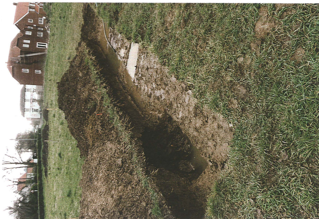
Plate 7: Trench 5: general view following excavation, showing catastrophic collapse of section excavated through ditch [503] in foreground, and ditch [507] being pumped dry, looking south-east.
