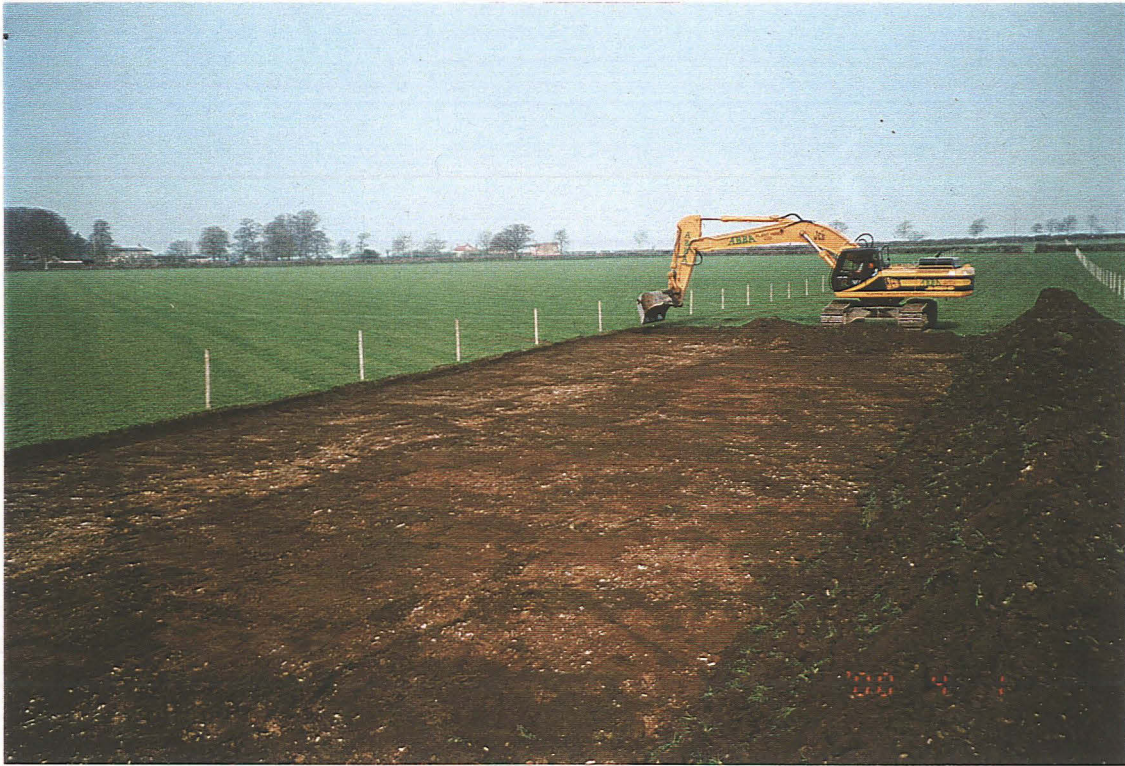
Plate 1: Plot 4. topsoil stripping in progress, note the modern plough scores, running diagonally across the easement, cutting into the subsoil. looking north-west.
