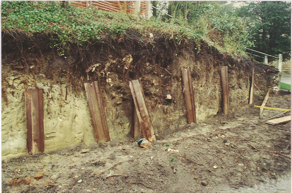
Pl. 6 View of the mixed clay material 1 overlying sandstone bedrock at the SE corner of the churchyard (looking east).
