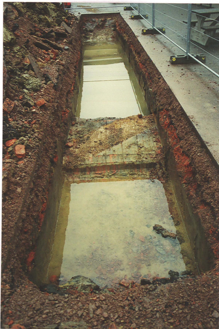
Pl. 6 Trench 2 after excavation showing flooding.
