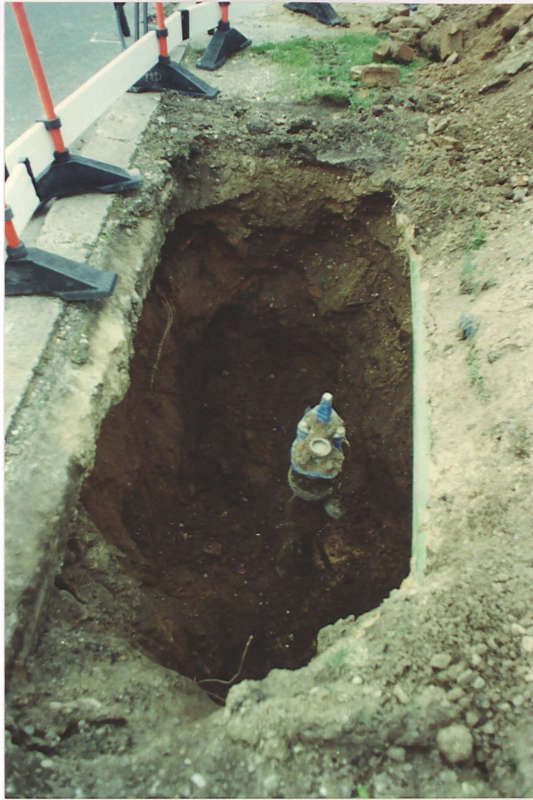
Pl. 1 Access hole alongside De Wint Avenue; many of the trenches remained within the backfill of earlier mains trenches.
