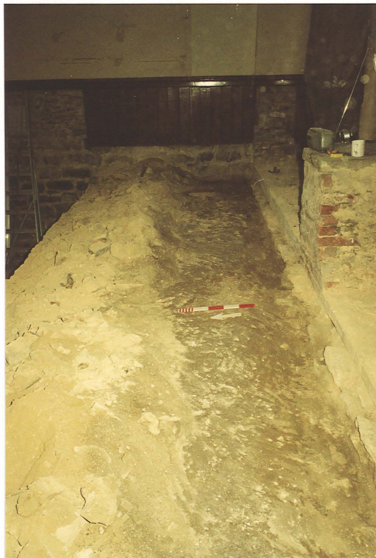
PI. 4 Foundation trench 14 along north side of north aisle wall 1, showing stone foundation 2. Looking east.
