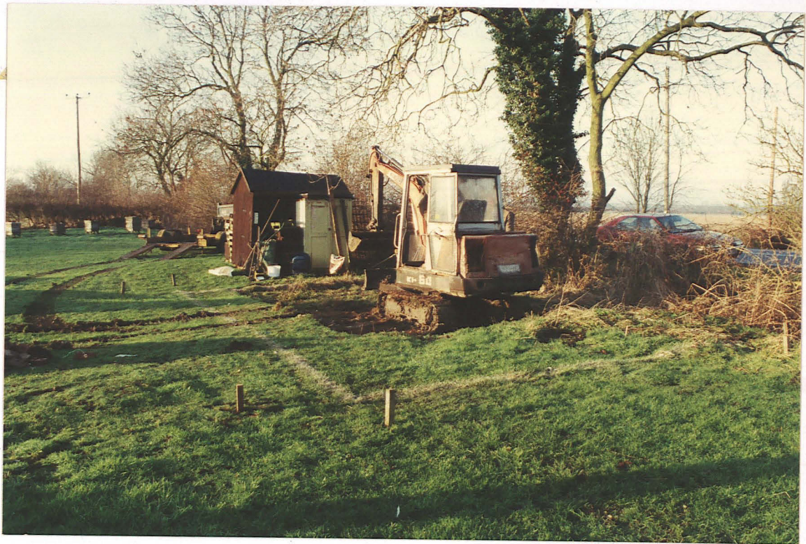
Pl. 1 Site of the new building (marked in white) beside Louth Road (looking SW).
