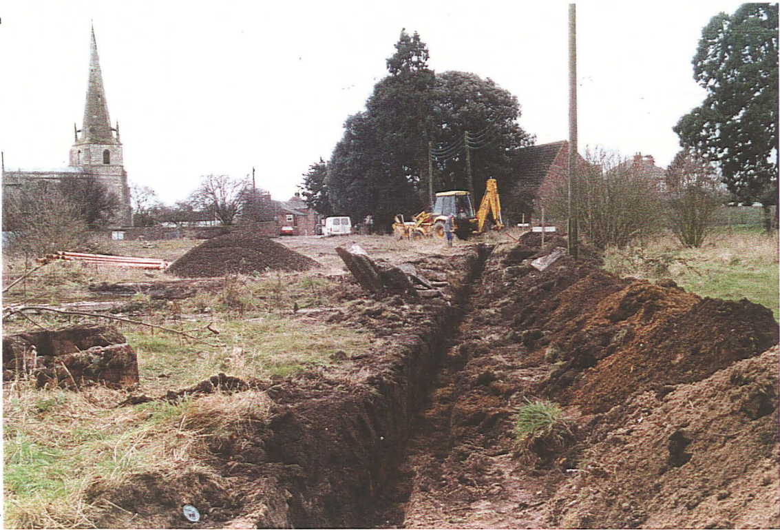
Plate 1: General view of the site, showing excavation of the main sewer trench (looking south-west)
