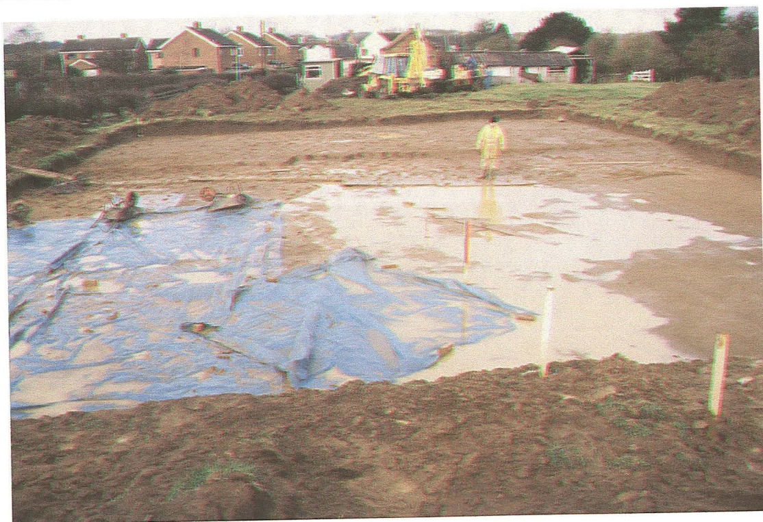
Plate 2: Serious waterlogging experienced during excavation - looking north-west
