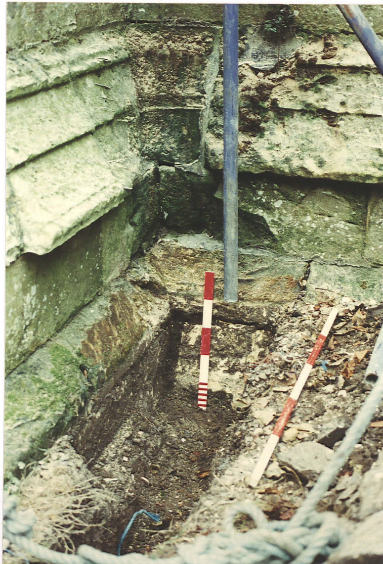
Pl. 5 Lower plinth at the SW angle of the tower (scales 1m and 0.5m).
