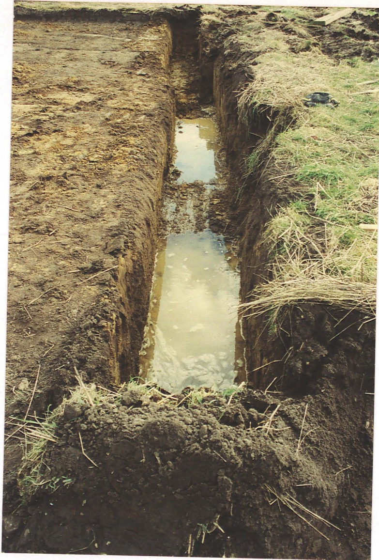
PI. 7 Footing displaying difficult ground conditions.
