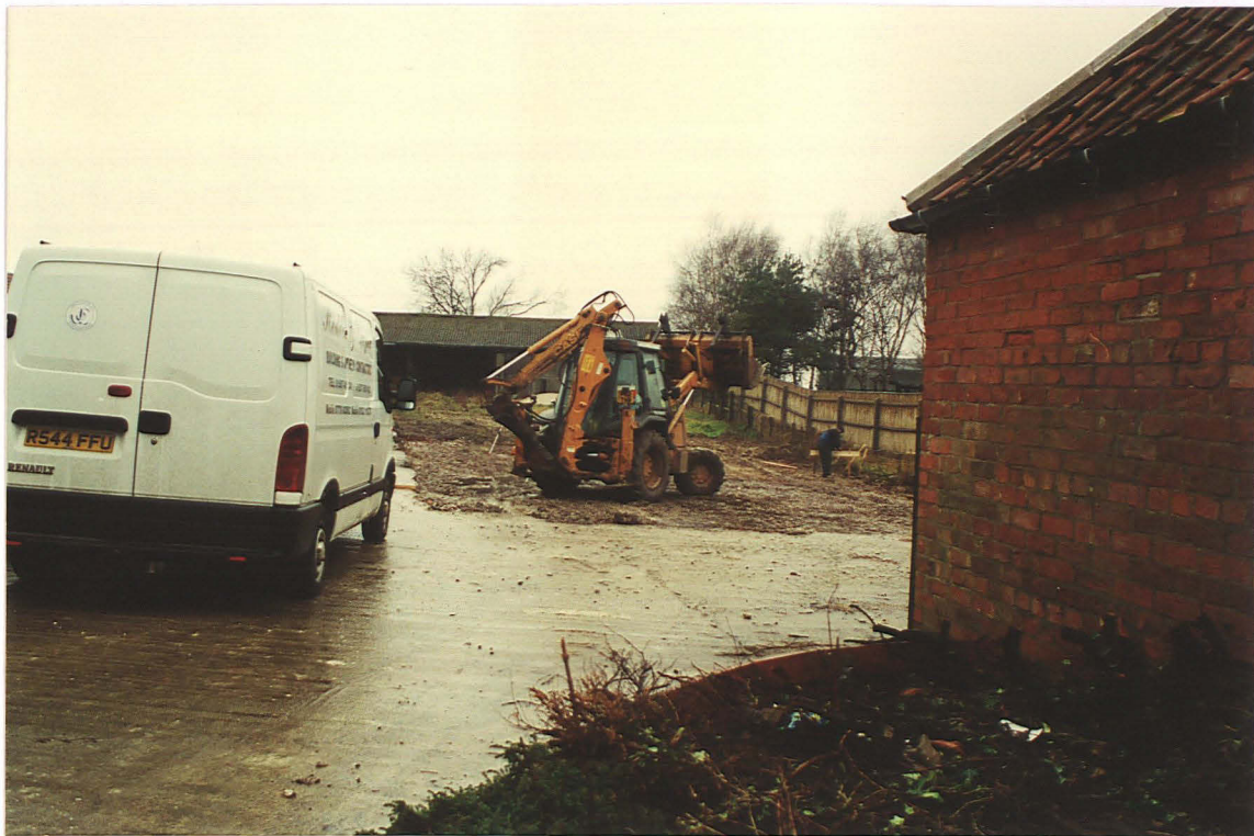
Pl. 1 The development site after removal of part of the concrete crewyard surface (looking NW).
