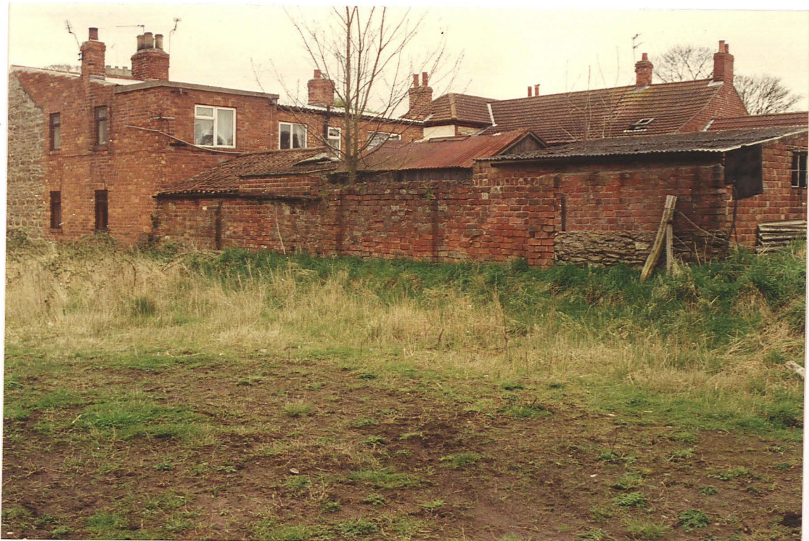
Pl. 12 Stonework in No. 72 High Street (left) and in the southern site boundary wall (looking SE).
