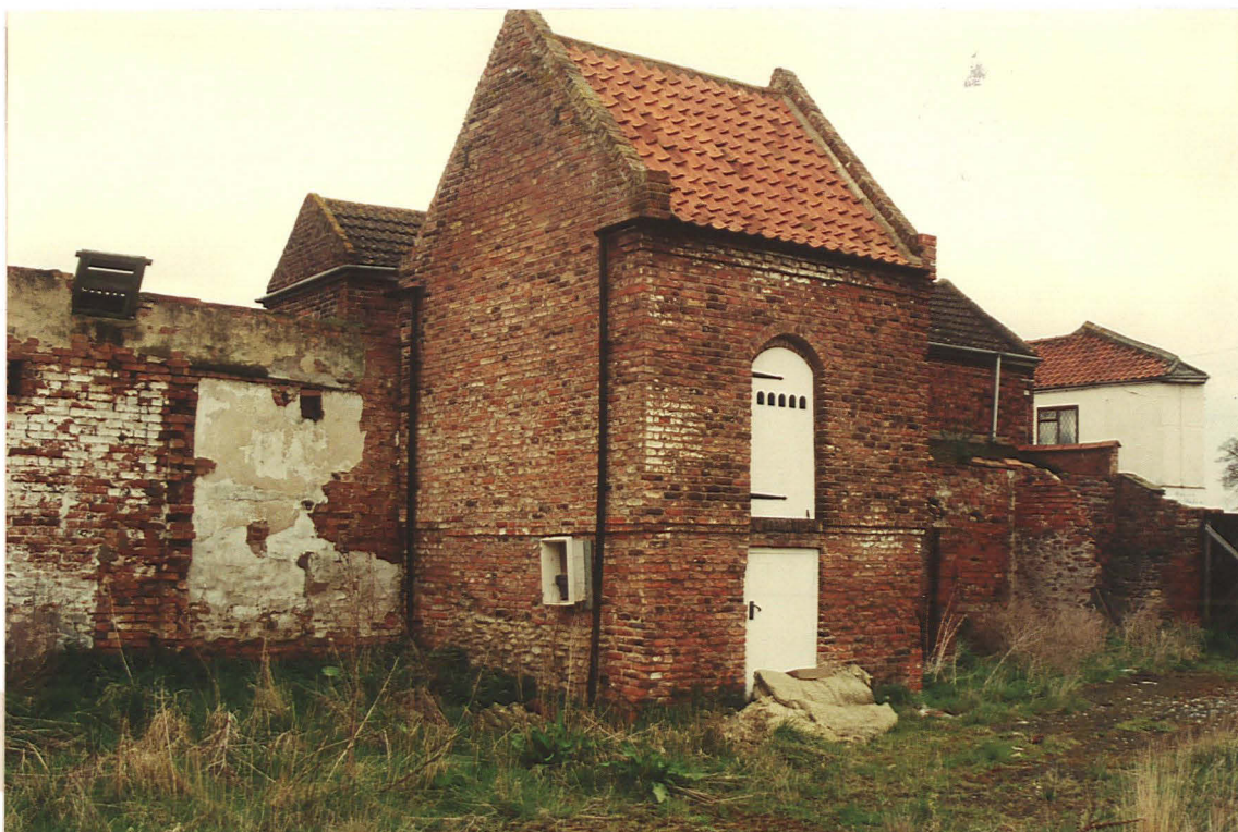
Pl. 2 The repaired early eighteenth century dovecote in the NE corner of the site, showing stonework at the base of one wall (looking NE).
