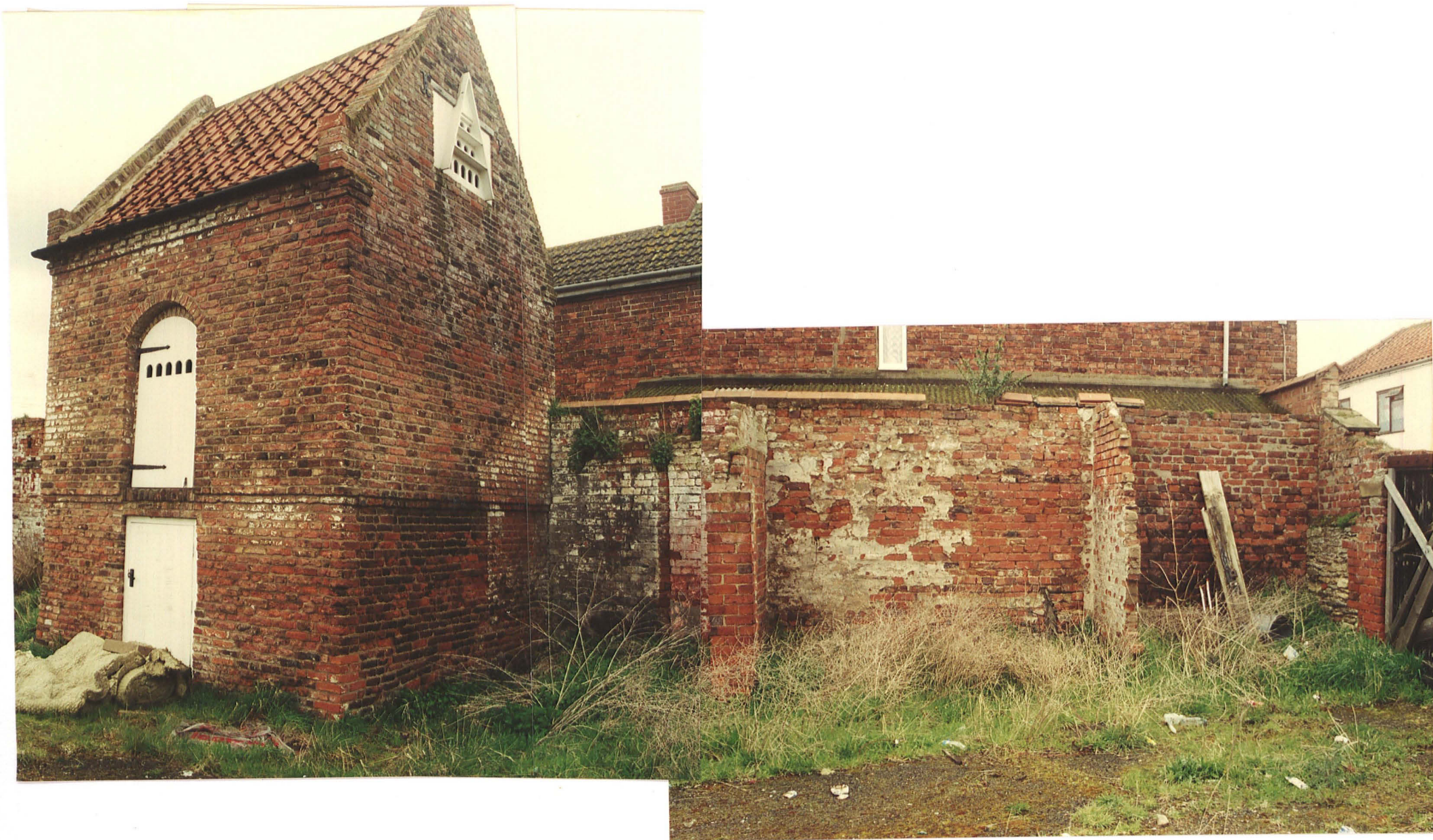
Pl. 3 Composite view showing evidence for removed buildings between the dovecote and the High Street frontage, with a short section of stone wall north of the entrance (looking north).
