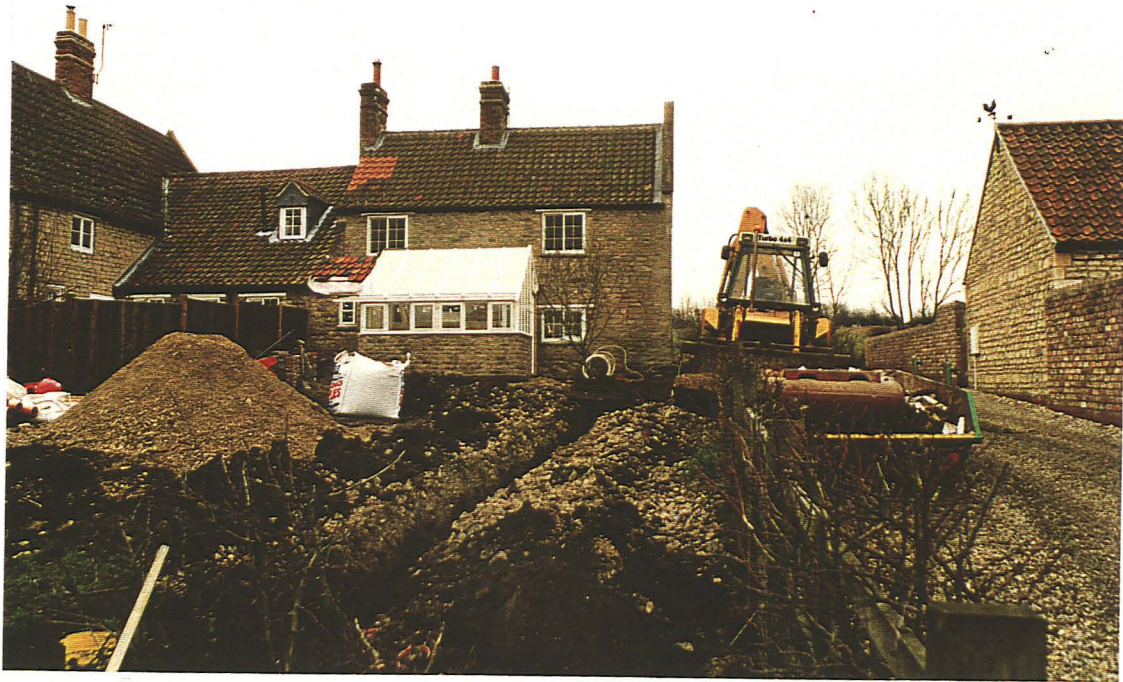
Pl. 1. Location of watching brief service trench, with Farm Cottage in background. Looking SE.
