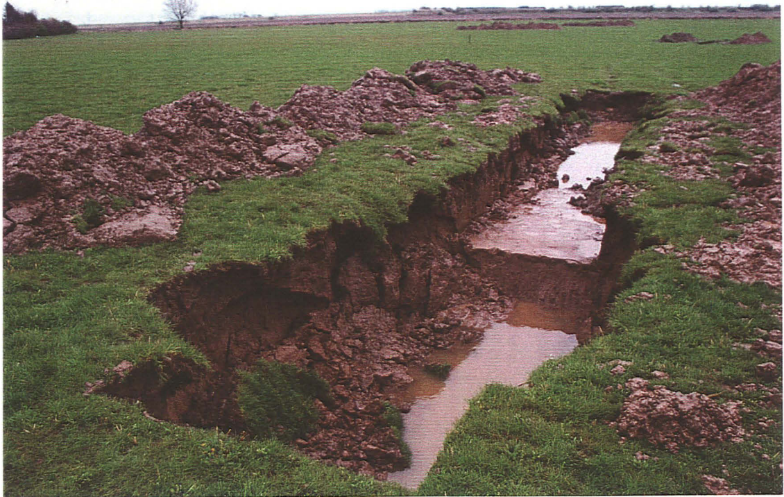
Plate 7: Trench 3, demonstrating the degree to which these sediments were prone to inundation and collapse, looking south-east.
