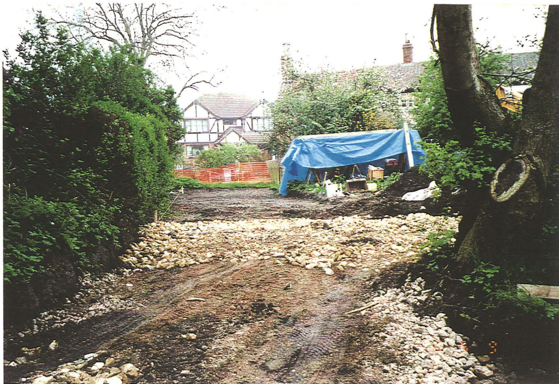
PI 1. Garage block excavations within rear garden of No. 4 Church Cottages, looking SW.
