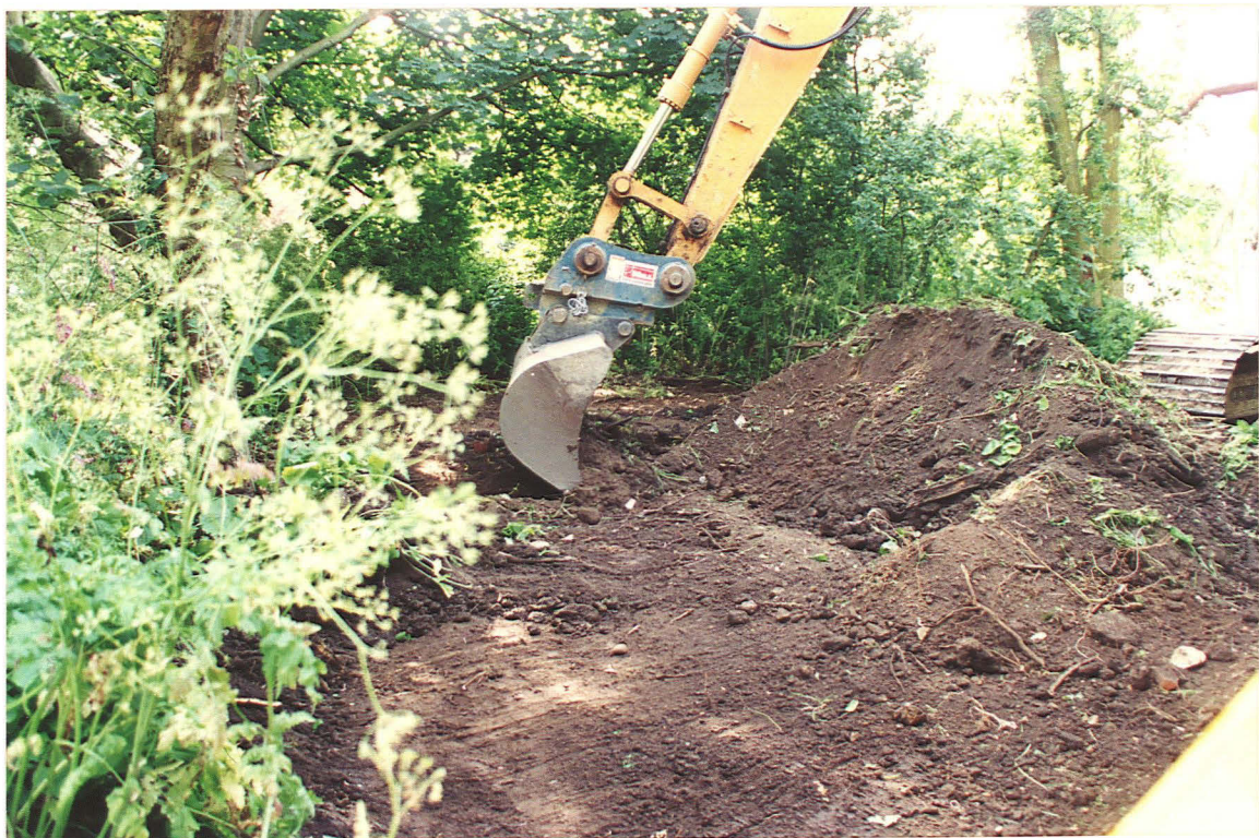
Pl. 2 Removal of topsoil from copse, next to Royal Oak Lane, to east side of raw access road.
