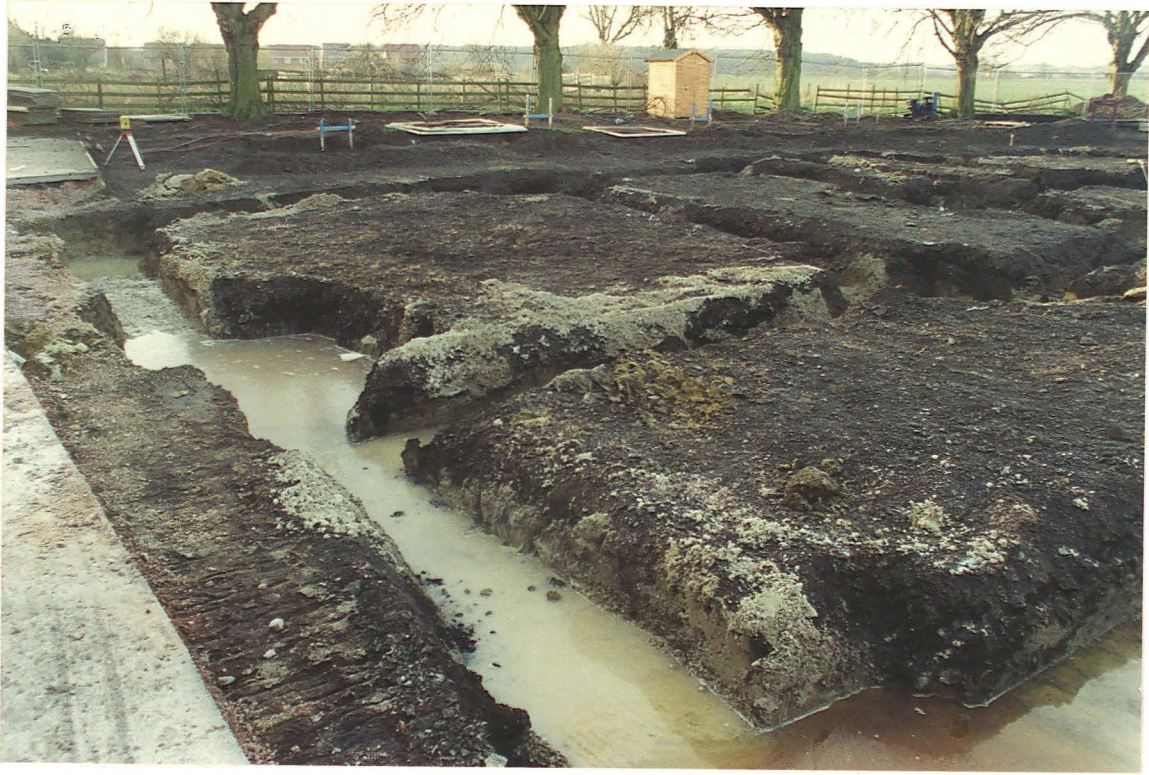
Pl. 11 Flooded foundation trenches during the watching brief
