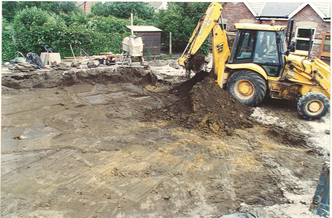
Pl. 4 Topsoil stripping in progress at east end of area, with natural yellow clay visible in front of JCB.
