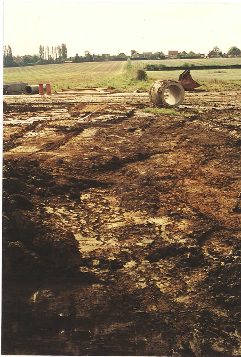
Pl. 3 Backfilled field boundary ditch (looking south along the surviving field boundary, towards Barrowby Road).
