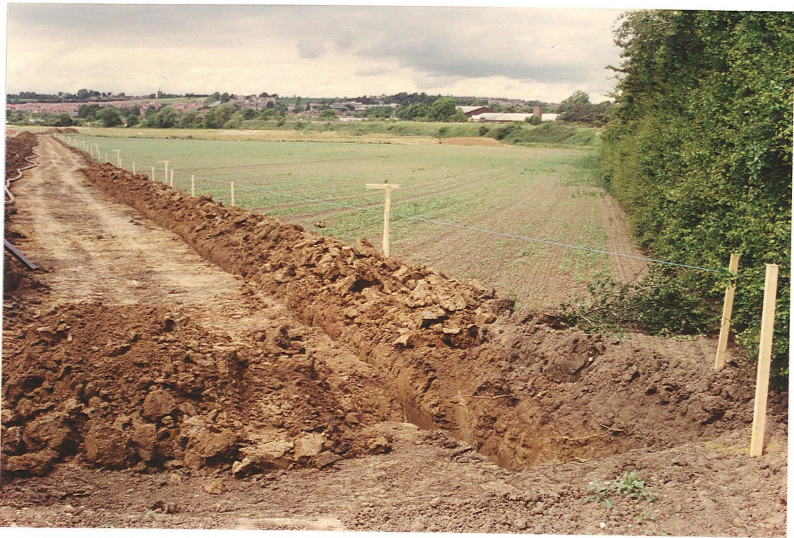
Pl. 7 The stripped easement, with part of the narrow pipe trench excavated (looking NW towards Gonerby Hill Foot).
