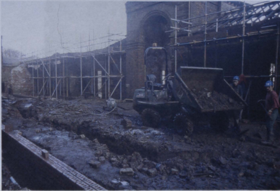
Plate 1 - General view of the development to the south of the existing workhouse buildings. The boundary wall is partially built and the foundation trench for the rear wall has been excavated
