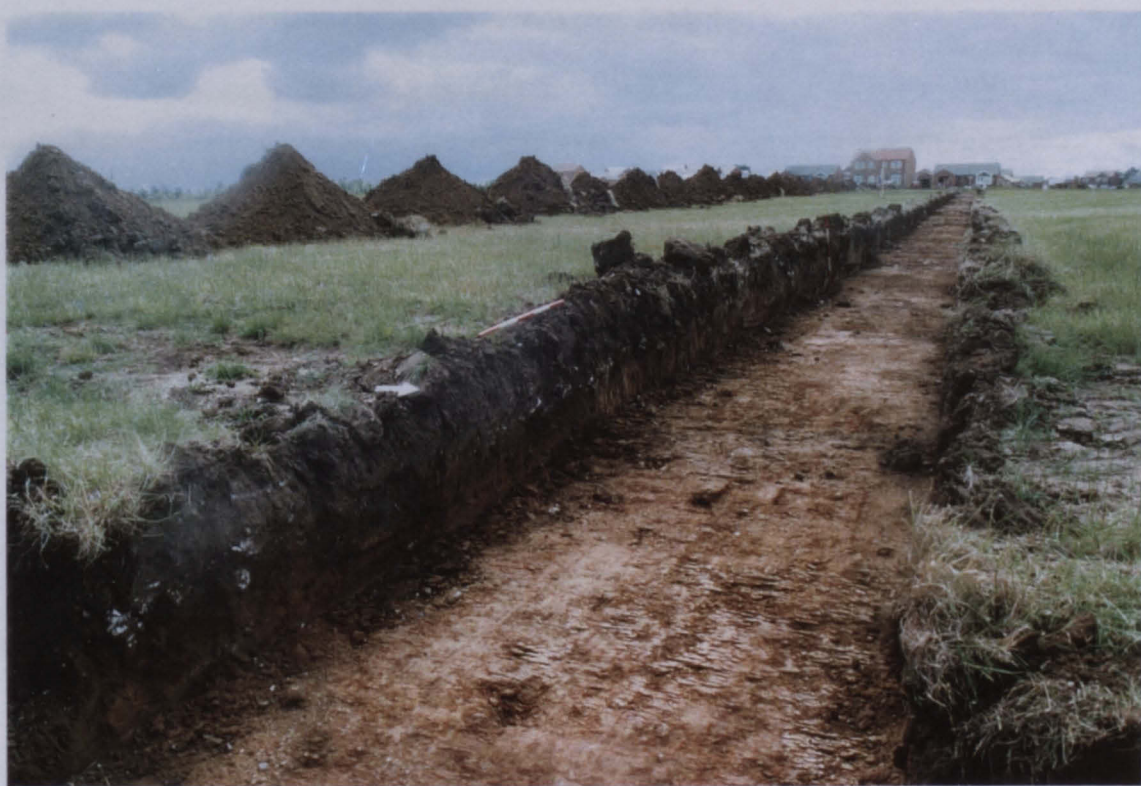
PI 8. Sewer trench in south field after initial excavation, looking west-south-west. Note rubble spread (044) in north-facing section. Vertical 1m scale shows westernmost extent of (044).
