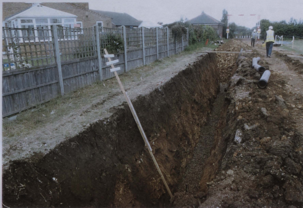
PI 1. Sewer trench excavations in north field. Looking north. Ditch [014] can be seen running along the east – facing section of the trench.
