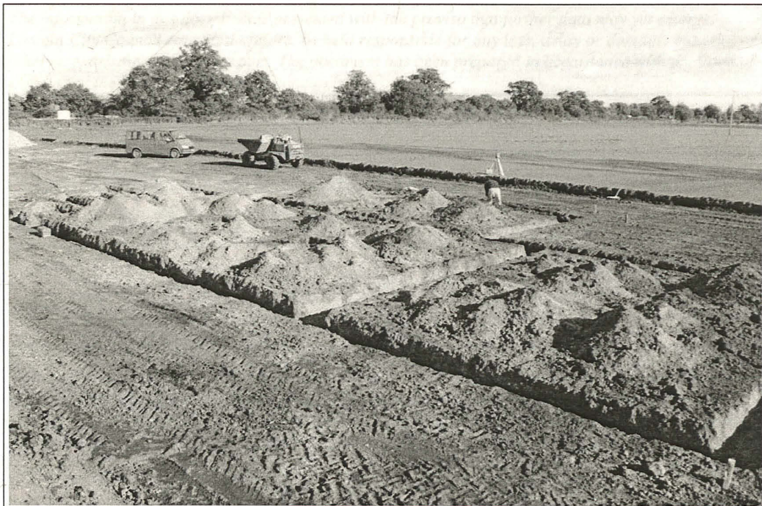
Plate 1: General view looking north-east, showing the excavation of foundation trenches for the clubhouse.
