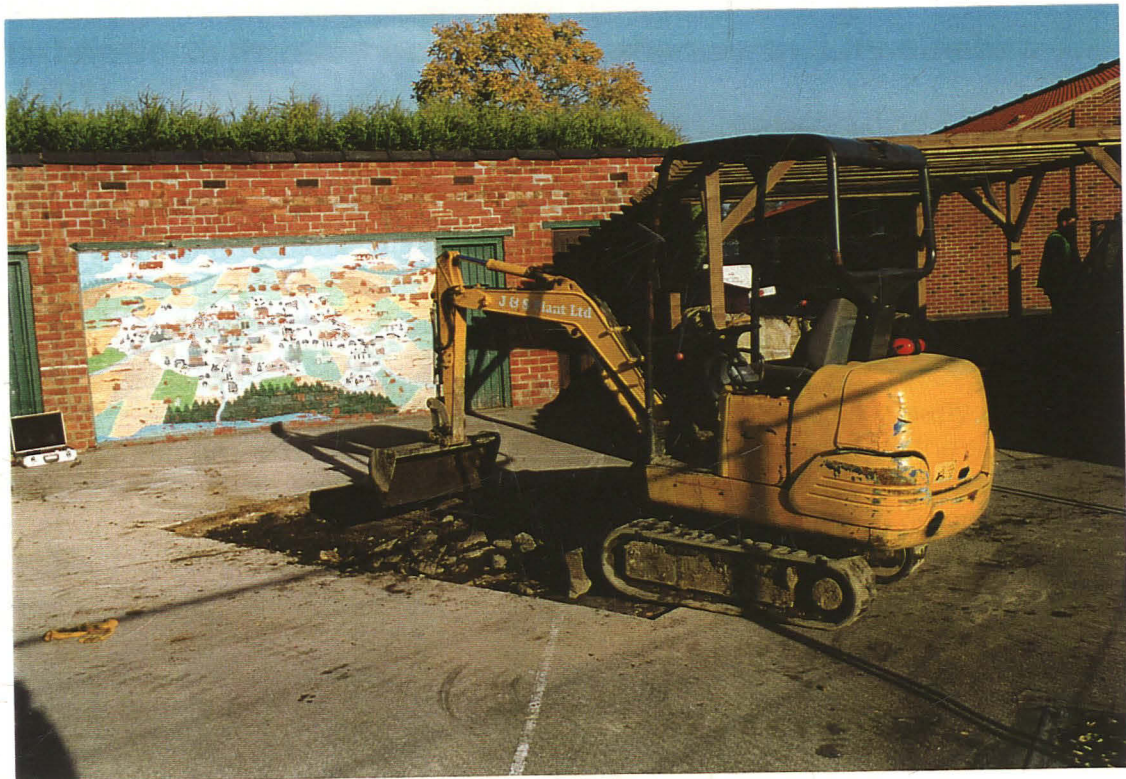
Plate 1: General view of Trench 1 during the removal of the playground surface, looking north.
