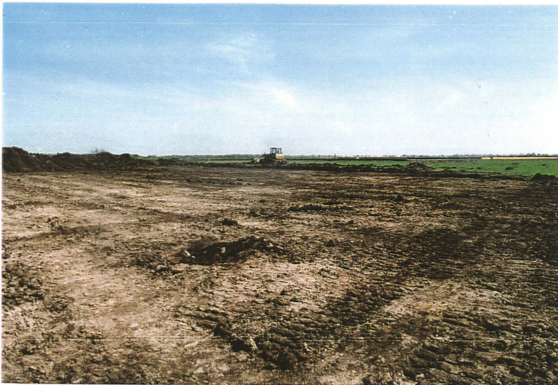
Pl. 1. General view of site, showing tracked bulldozer stripping topsoil and subsoil, looking SE. Treebole [006] is visible in the foreground as a dark area.
