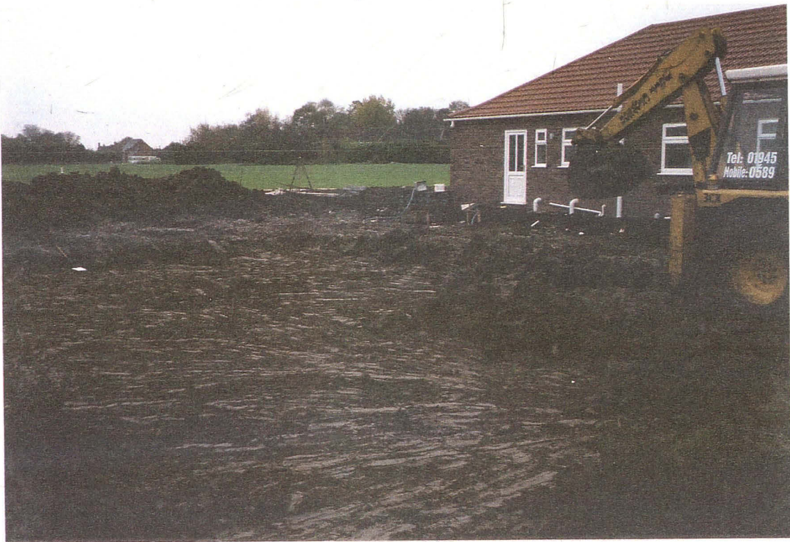
9.2.1 Plot 6 showing the machine stripped surface for the concrete raft foundations of the bungalow
