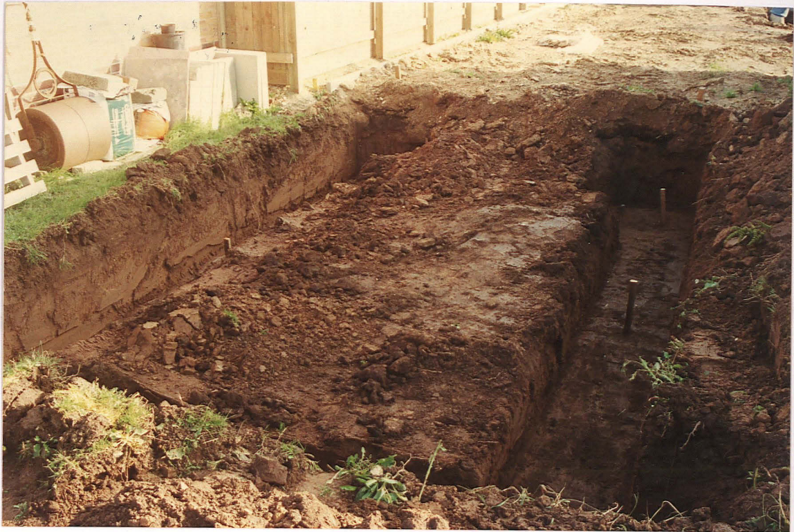
Pl. 1 Foundation trenches for the garage, Plot 5 (looking east towards Drury Lane, with the boundary of Plot 6 (formerly Plot 10) to the left).
