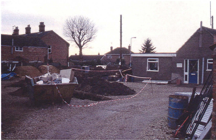
Plate 1 General view of the site looking southwest, with Trench 1 in the foreground.
